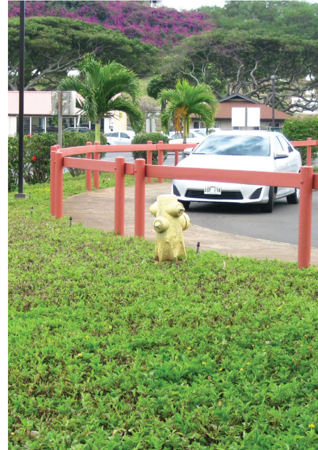
Fire hydrant at Church circle.
