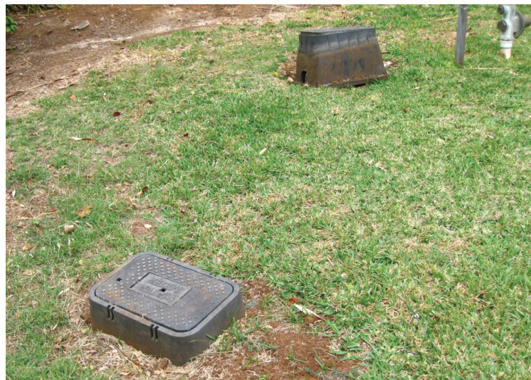
Existing water meters behind Church.
