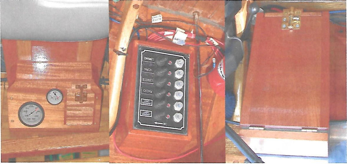
Figure 14, 15, & 16: Views of fuse block and circuit breakers on transom; gauges on port side.
