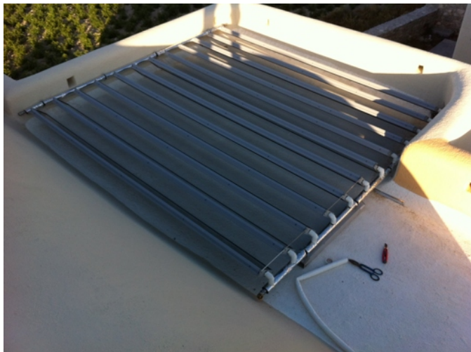
Panels can be turned around in summertime in order to avoid excessive water heating when not habited.
