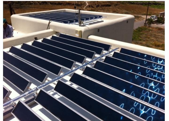
All roof areas are covered by 20 +9 solar panels (3.0/2.0 m) with high efficient selective surface ( a=95\% e=5\% )
