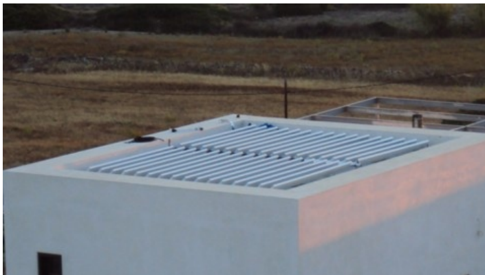
The solar panels have a very low (20 cm) 'high profile' and are not visible from the street level.
