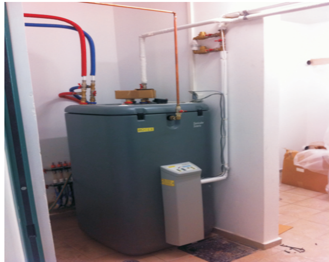
The non-pressurized solar water storage tank 500 L is well thermoinsulated to keep a mean temperature of 55-60°C.
