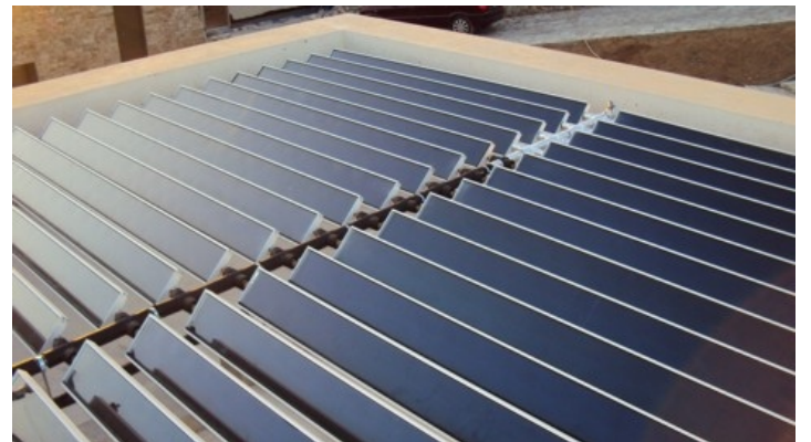
Panels can preferably be arranged in symmetric arrays covering of the whole of the available roof area.
