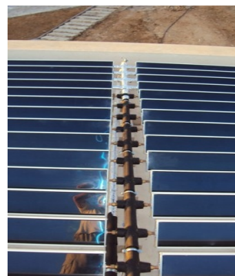
The hot water collector pipe must be higher to air vents.
