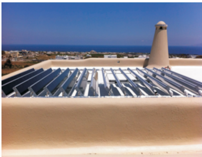
Panels are not affected by strong winds due to its free space the angle can easily be adjusted by turning in groups of four.
