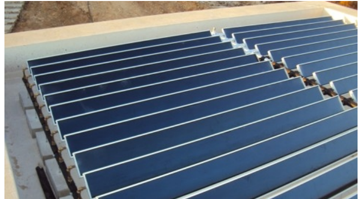
The solar panels are equipped with a 'blue' selective highly efficient al. surface ( a=95\% e=5\% ) welded on copper pipes.
