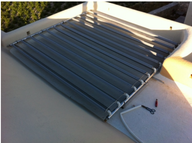
Panels can be turned around in summertime in order to avoid excessive water heating when not habited.
