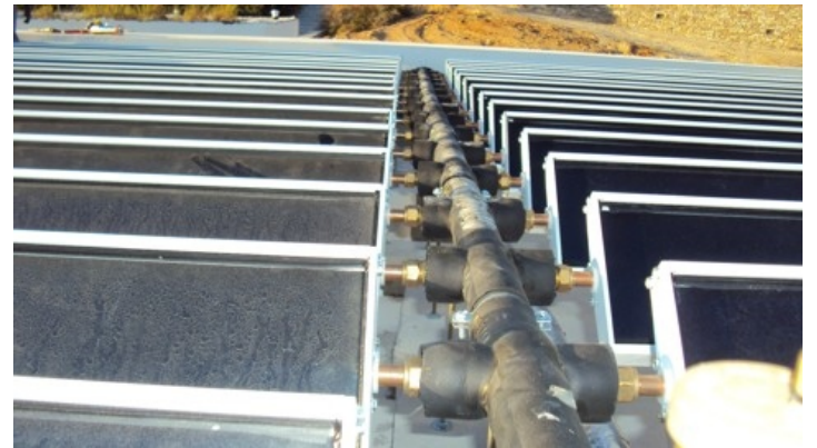
Panels can preferably be arranged in symmetric arrays. The hot water outlet pipe must higher than the inlet pipe.
