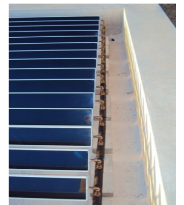
Cold water distributor pipe is mounted lower with elbows.
