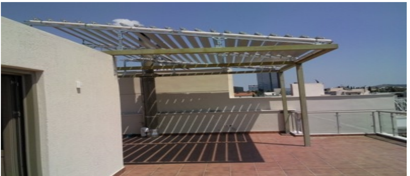
Installation as shadowing pergola for floor heating system, hot water and pool heating.
