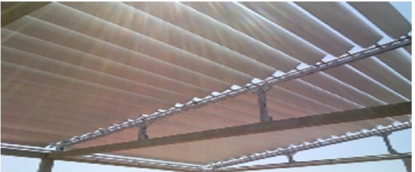
Installation as shadowing pergola for floor heating system, hot water and pool heating.
