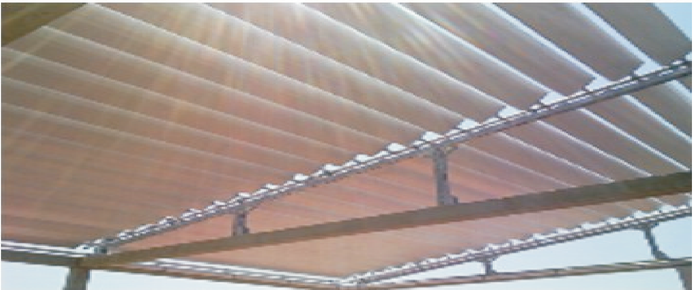
Installation as shadowing pergola for floor heating system, hot water and pool heating.
