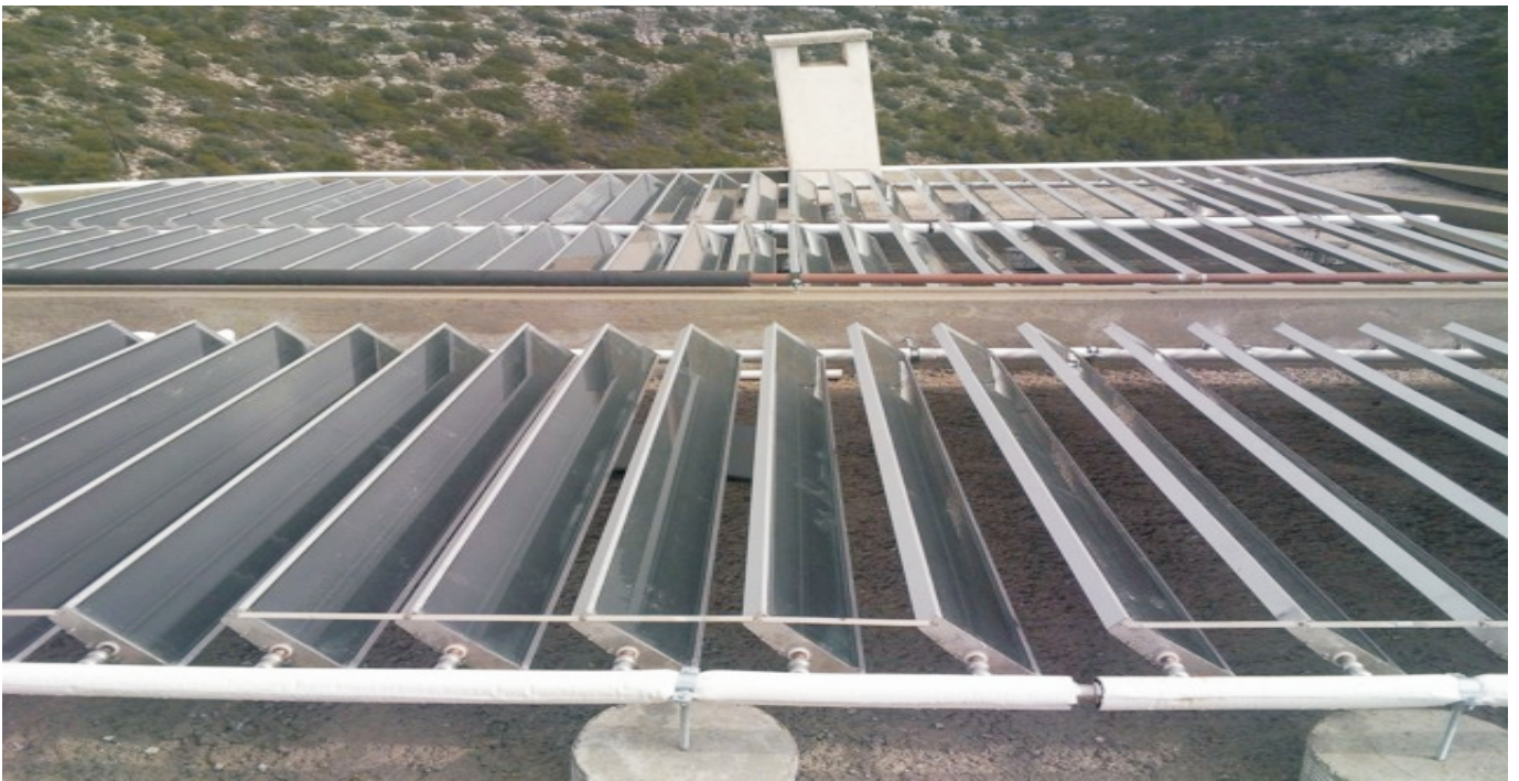
Installation on flat roof for central floor heating system, hot water and pool heating.
