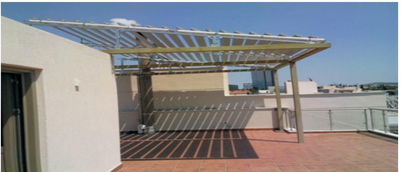
Installation as shadowing pergola for floor heating system, hot water and pool heating.
