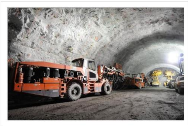
Loading a topheading round with a Sandvik T11A jumbo in the foreground
