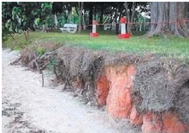
Figure 3.10. Coastal Erosion at East Coast Park, Singapore
