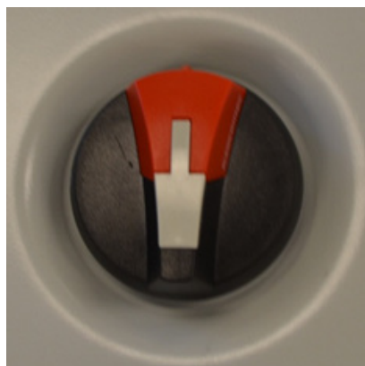
DC disconnect switch ON position
