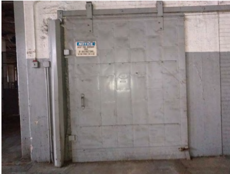
1. Gray metal fire door.
