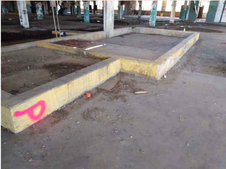
26. Yellow concrete floor bumpers.
