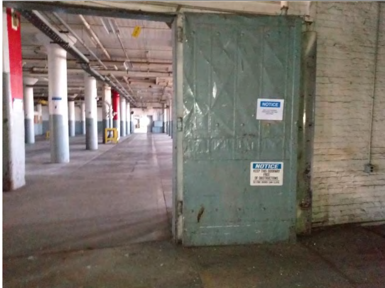
11. Gray metal fire door.
