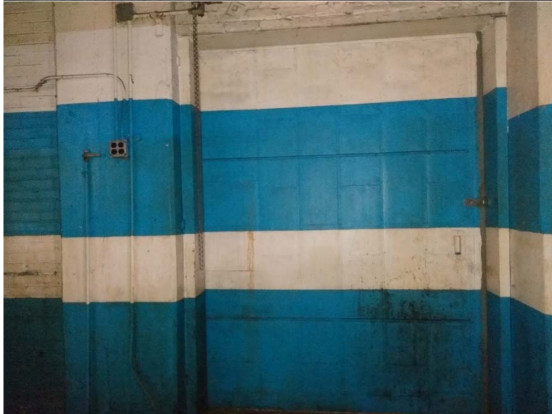
2. Blue and white on metal fire door, as well as concrete column and brick.
