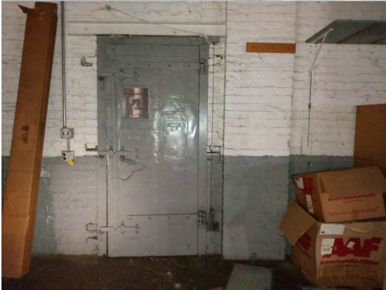
5. Gray metal fire door.
