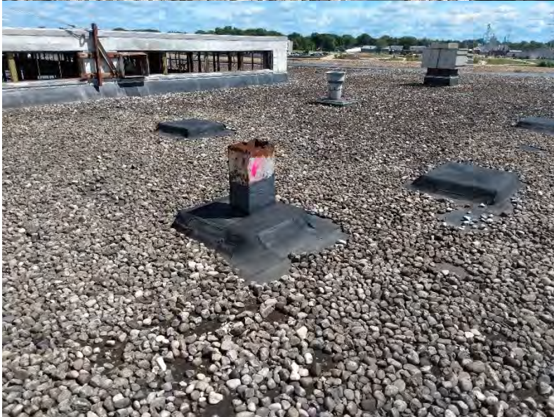
32. Gray metal on vent on rooftop.
