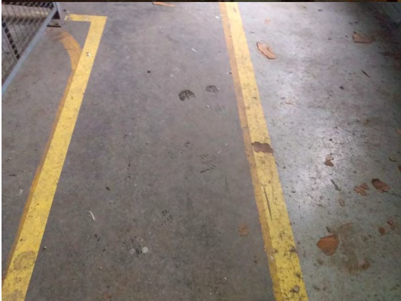
6. Yellow on concrete floor. *The older darker shade of yellow was positive, while the brighter, newer was not. Where the two overlapped still tested positive for lead, due to the underlying layer.
