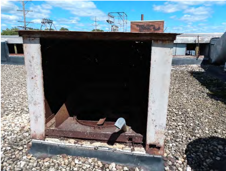
31. Gray metal on machine on rooftop.
