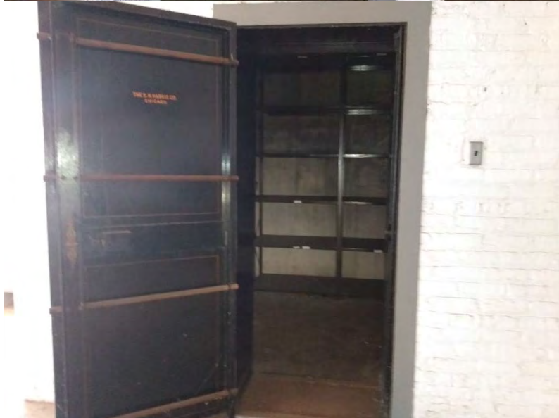
14. Safe door, frame and green on the interior walls.
