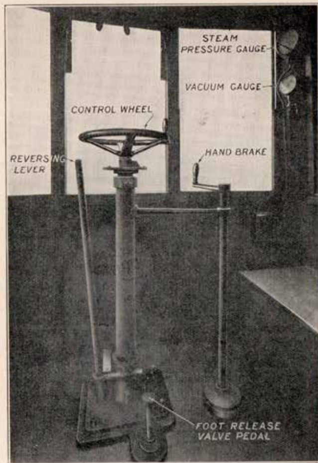
Showing the Car Controls at Rear End.
