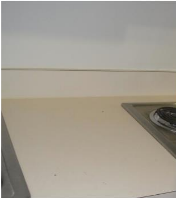
Figure 7. Kitchen counter wider than 12", Missing a GFCI outlet.
